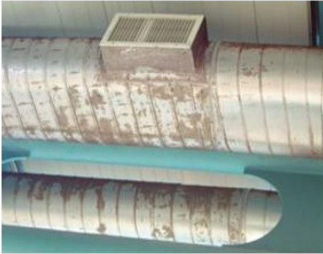
Corroded Air Handling System
